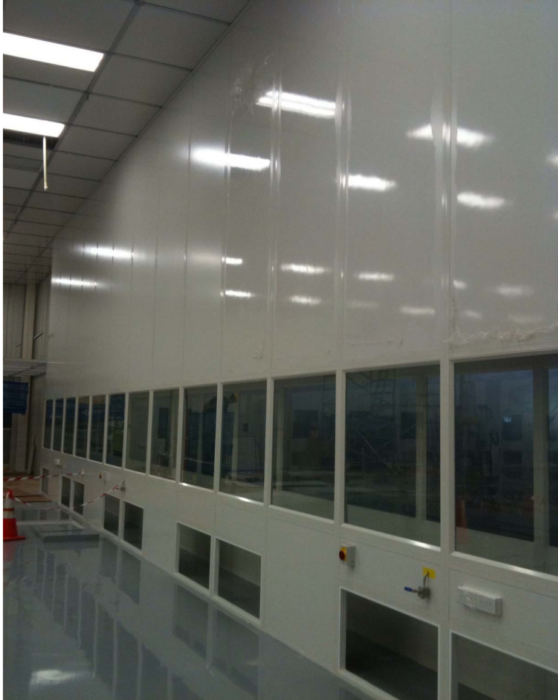
Figure 10: SFS2000 System 8.5m Height with Continuous Window and Return Air Grille Opening
