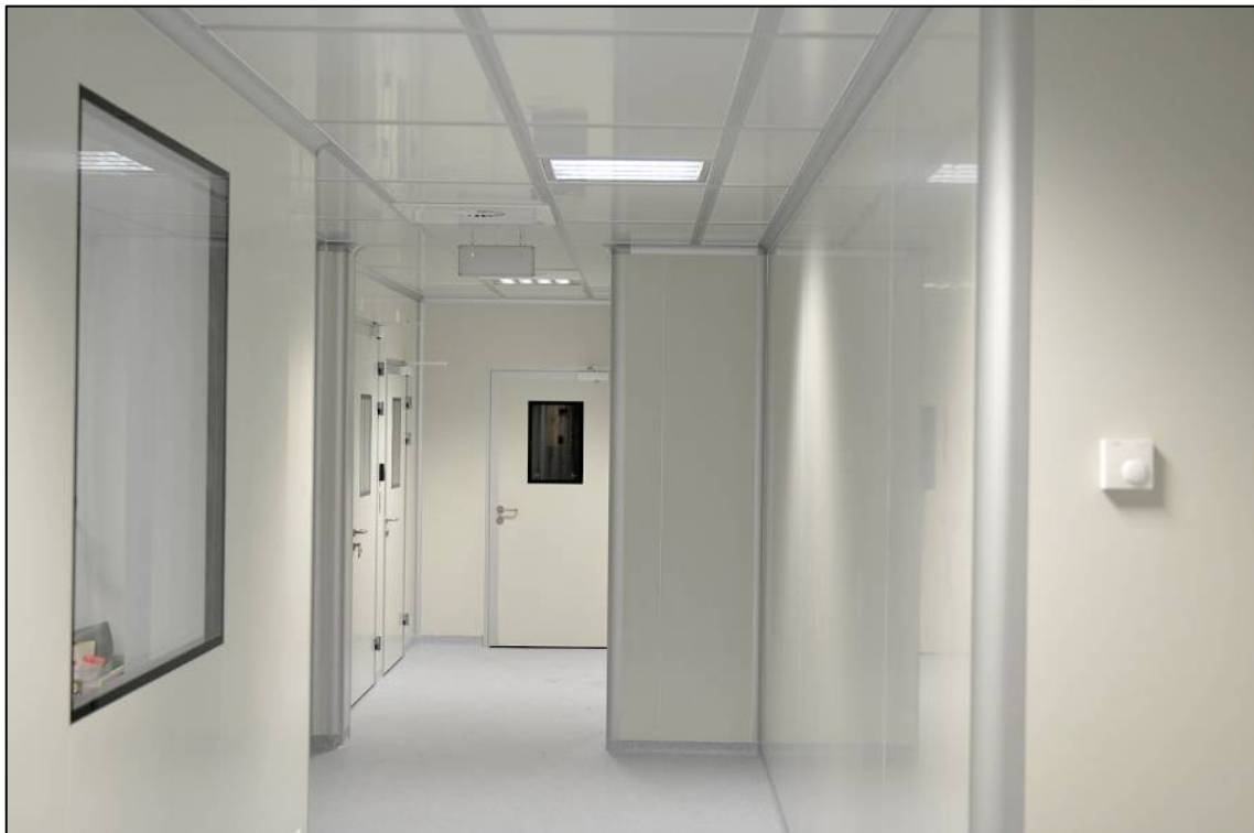
Figure 13: GMP50 Systems Typical Appearance
